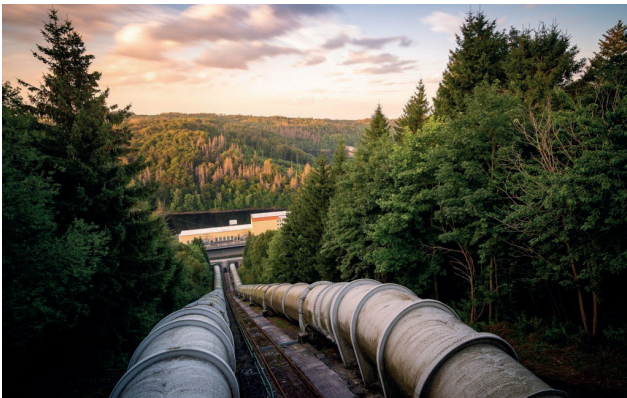
Penstocks of a hydropower plant
